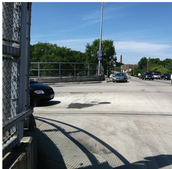
The narrow sidewalk on Harlem creates a hazard for pedestrians entering and exiting the Blue Line station.
