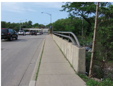
Existing Condition of sidewalks on the Des Plaines Avenue Bridge.
